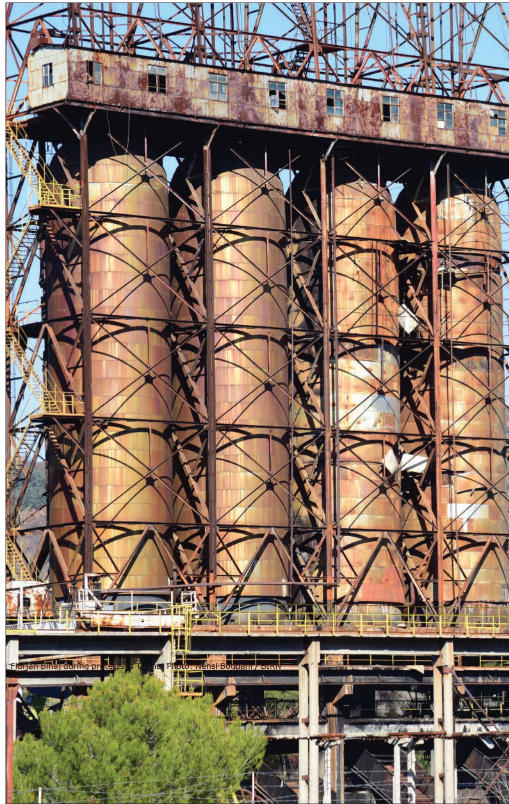
Demolition of the refinery, where the Shijaku company says it will build a solar park. Photo: Nensi Bogdani/BIRN
